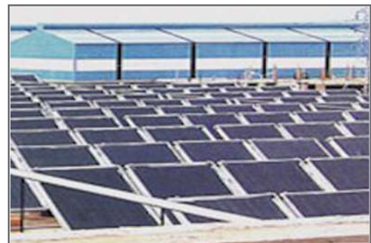
Fig 3.15: Solar Panels to trap solar energy
